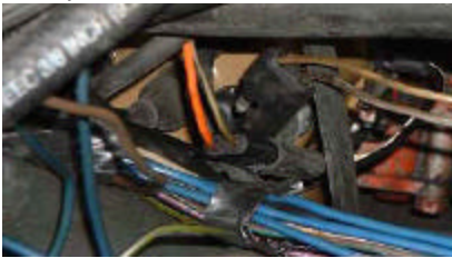
This one shows the spliced distributor connector connected, and the old Chrysler Electronic Unhooked.
